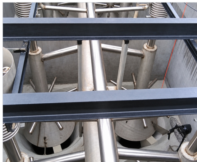
Installed multi-vessel arrangement with common distribution header.
