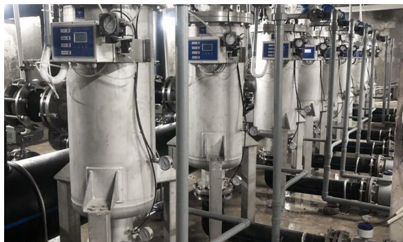
Parallel filter bank for higher-flow service.
